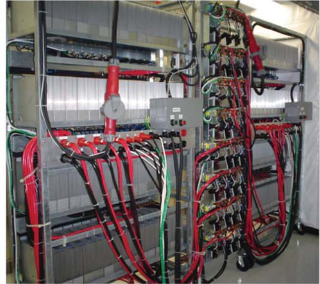
Rear view of Burn-In Cart and Inverters
