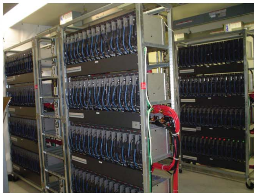
Front view of Multiple Burn-In Systems
