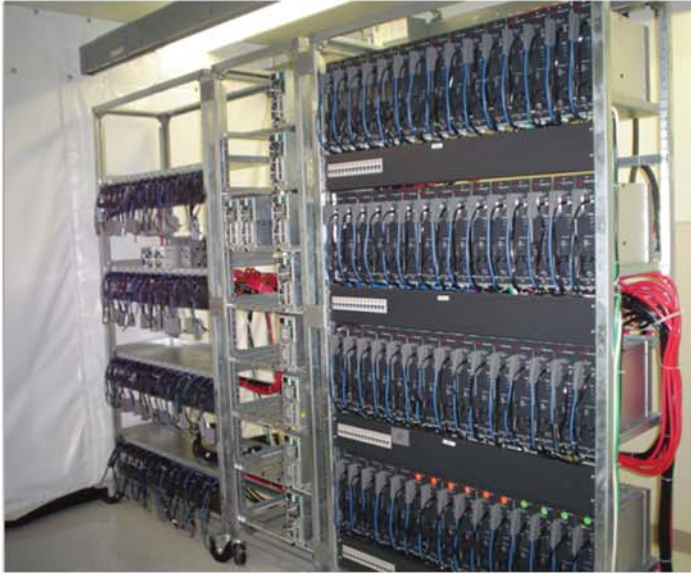
Front view of Burn-In Cart and Inverters
