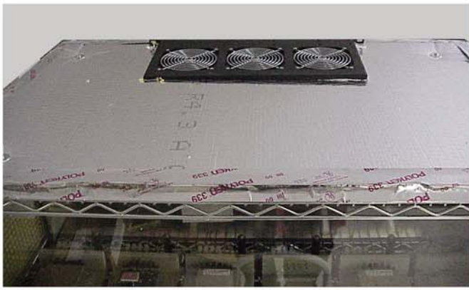
Heat Exhaust Fans on Top of Cart
